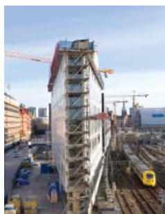
Emerging at Norra Bantorget is Skanska's Swedish answer to New York City's historic Flat Iron Building: 14,000 sq. m (150,000 sq. ft.) of modern, flexible office space. A more central location is hard to find in Stockholm.
